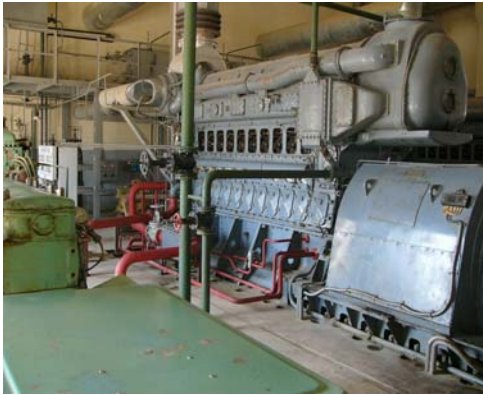
Figure 4: Old Soviet-era generator
