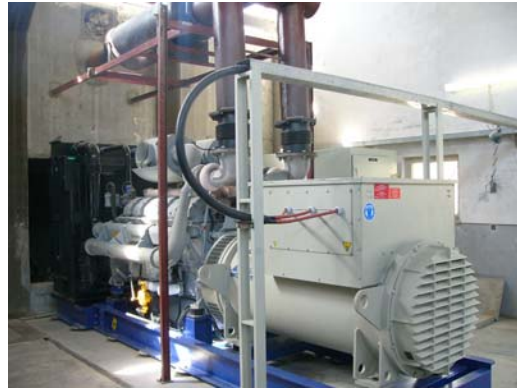
Figure 5: New USAID-supplied generator
