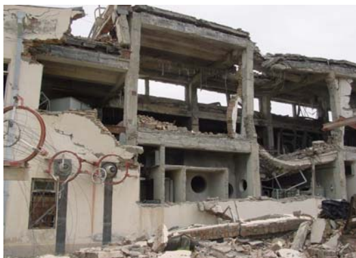
Figure 2: Transmitting station before repairs
