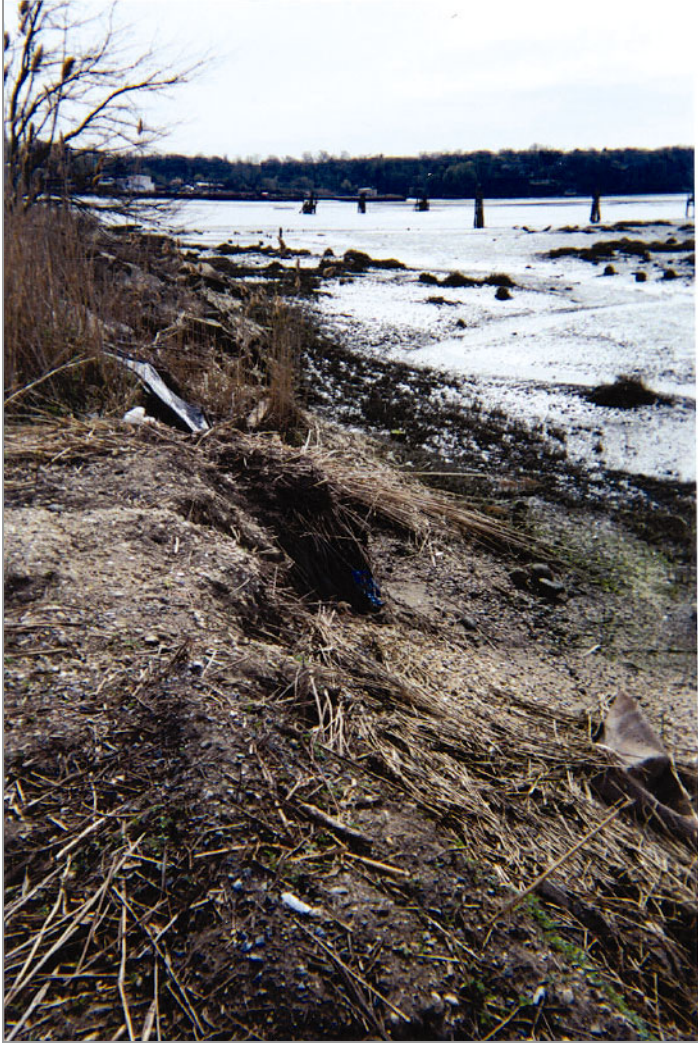
Photograph 7: The northern most shoreline of the Bar Beach Lagoon, which is adjacent to the Bar Beach parking lot. Note the sharp slope containing rubble and debris. The material that makes up the shoreline is a mixture of loosely consolidated soil and rubble/debris, which makes the shoreline moderately unstable.
