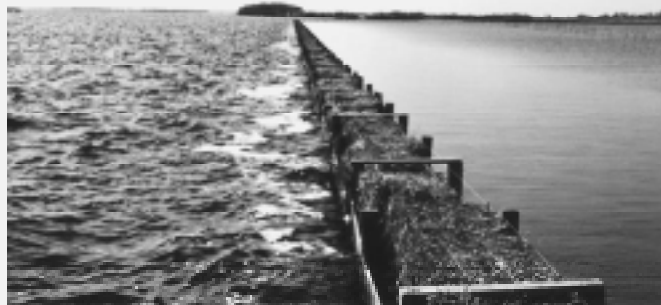
The impressive effect of wave-damping devices is best shown in this photo. While water to the left of the fence is fairly turbulent, water on the right is calm, thereby minimizing erosion.
