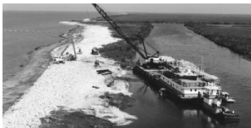
A barge-mounted drag line crane transports limestone rock from the loading barge to an articulated dump truck on shore. More than 13,000 tons of rock are being used at Point Au Fer.
