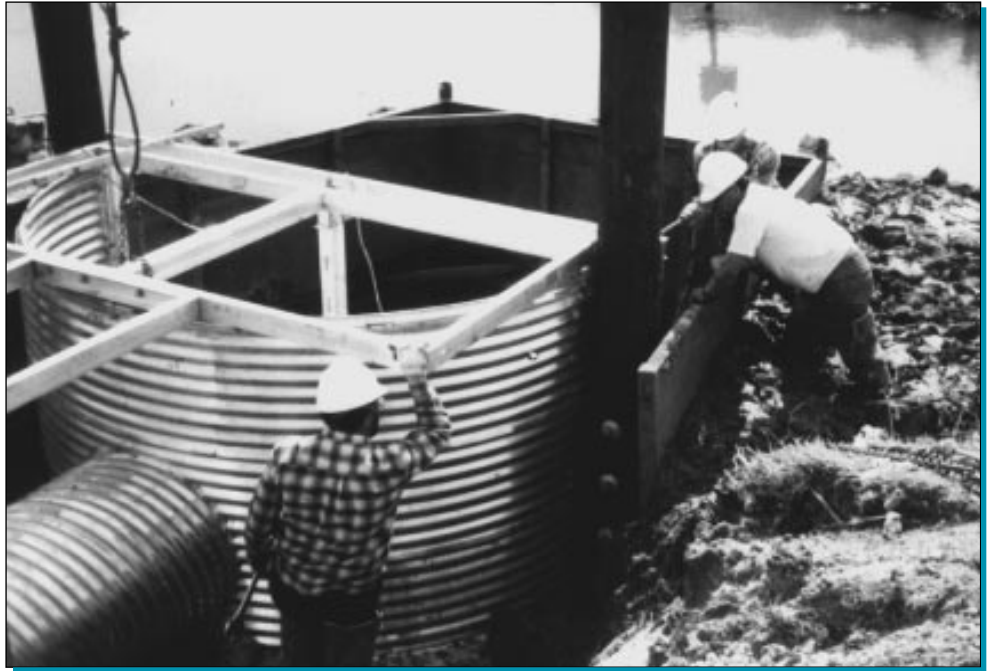
Workers install one of three double-barrel corrugated aluminum pipes at the East Mud Lake Project. Each pipe has a variable crest weir inlet section with a vertical slot.
