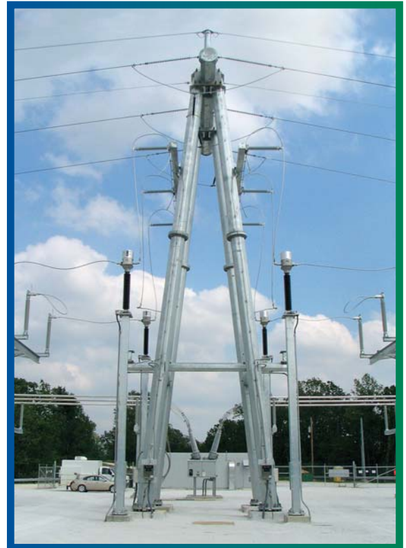
THE NEW HILLTOP INTERCONNECTION NEAR SILVER HILL, ARKANSAS, ADDRESSES REGIONAL TRANSMISSION CONCERNS.
