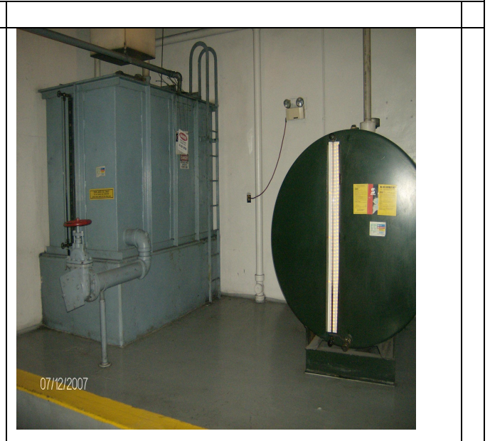
Illustration 3. OIG’s unannounced observation of oil disposal. Logbooks were up to date, and we found no signs of leakage.
