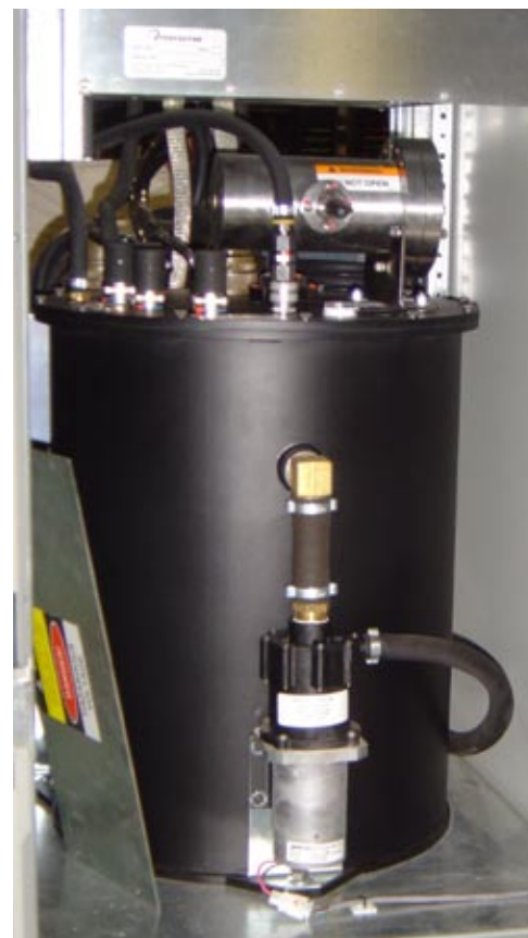
Figure 1. Flywheel uninterruptible power supply (UPS)
