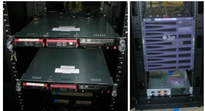
Figure 2. Servers modified to accept 380V DC
