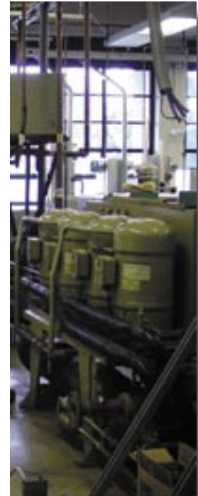
Figure 1. Hands-on HVAC training facilities at Laney College
