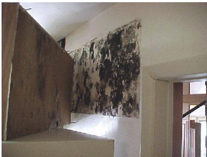
Figure 2. Some mold is hidden from view, such as the mold shown in this image, which was discovered when cabinets were removed from a wall (Photo courtesy of Mike McNickle)
