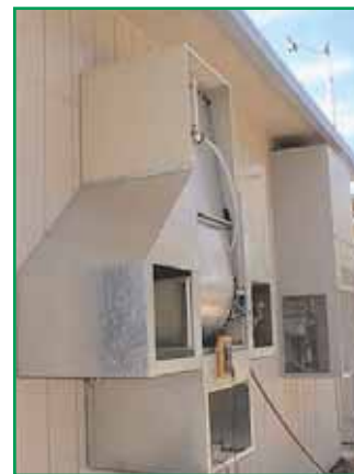
Figure 1. This HVAC system was designed for the relocatable classroom study.
