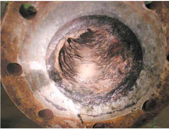
Corroded Cooling Water Line
