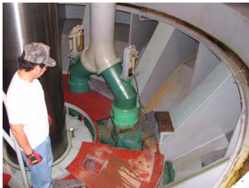
Vacuum Breaker Piping
