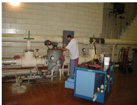
Main Cooling Water Piping
