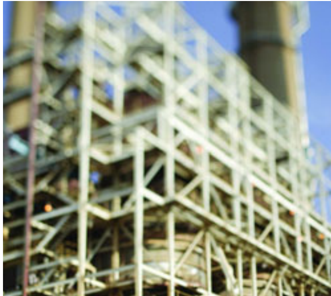
A scrubber at Paradise Fossil Plant
