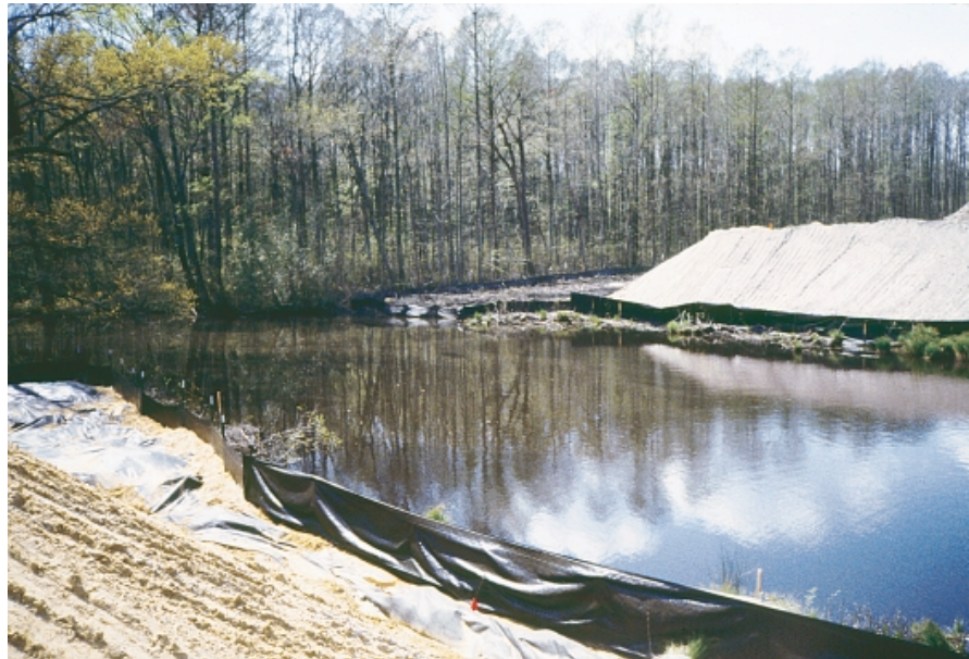
Figure 29. An example of forested wetland loss in Virginia, 1998. Trees have been cleared and the area filled for bridge construction.
