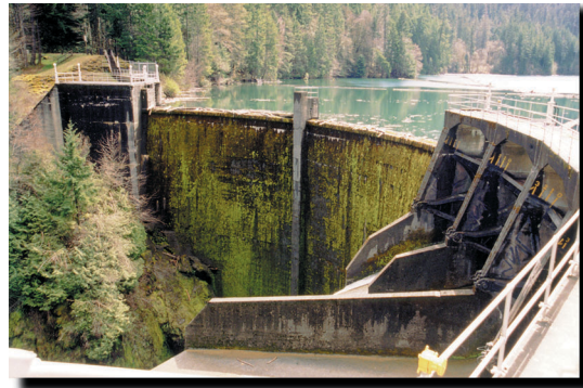
Safety of dam modifications consists of correcting identified structural deficiencies. These deficiencies could lead to a failure, resulting in uncontrolled releases of stored water that would place downstream populations and resources at risk (photo by BOR).
