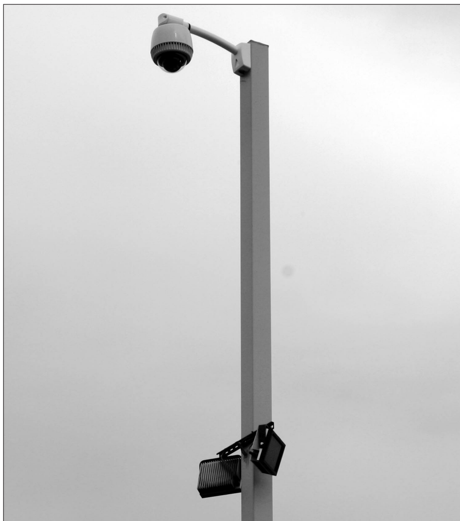
Figure 12: Security Camera and Infrared Motion Detectors
