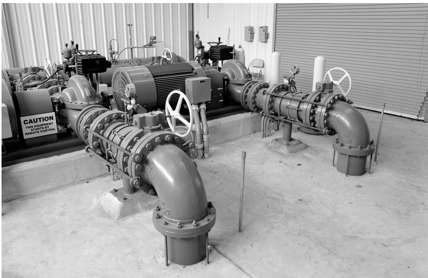
Figure 7: Pump Operated through Remote Automated Systems
