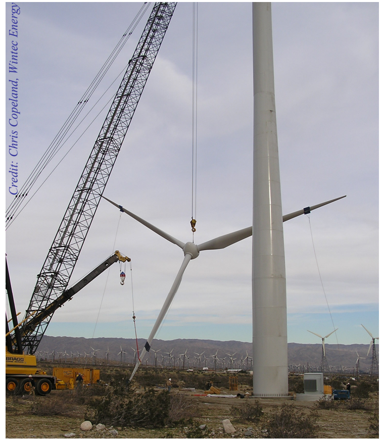
A key person on the wind farm construction team, a crane operator lifts the blades onto a wind turbine.
