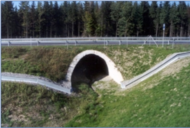
Figure 14. Arch culvert on German Highway B-30, with rail for amphibians and fence for larger wildlife.
