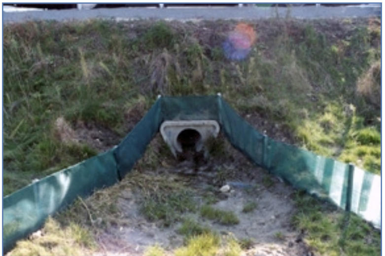
Figure 13. French pipe culvert for small mammals and amphibians.
