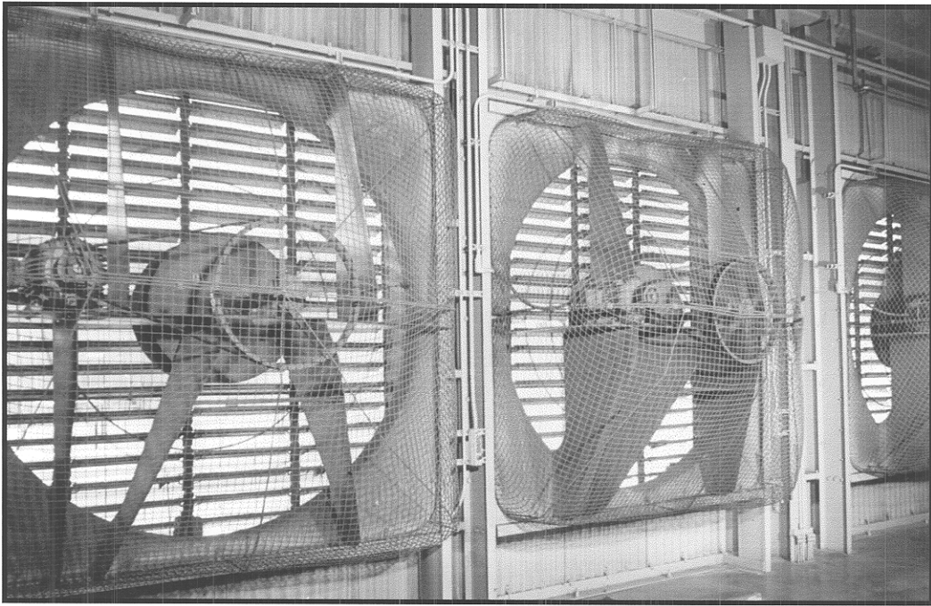
Photograph 5: Six-foot diameter fans were installed in Colex Building 9201-5 in 1956 to increase ventilation and thereby reduce airborne mercury concentrations in operating areas (Photo 102455 courtesy of the Y-12 Plant).
