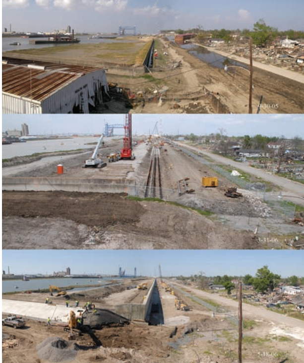
New Orleans, LA—Work progresses on repairs to the 9th Ward Levee that was damaged by Hurricane Katrina. FEMA provided Public Assistance funds to repair New Orleans Levees to Category 4 status. (Marvin Nauman/FEMA photo)
