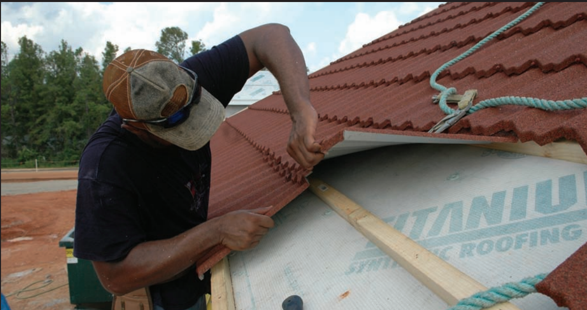
Gulfport, MS, August 15, 2006—Contractors are now replacing the temporary blue roofs with permanent roofs. Hurricane Katrina destroyed countless roofs along the Mississippi Gulf Coast. (Mark Wolfe/FEMA photo)
