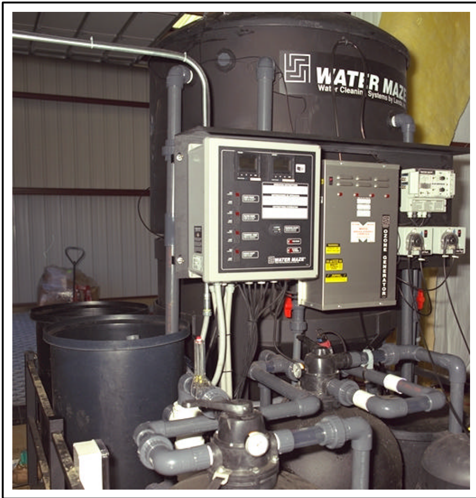
Figure 1. Landa System in Building 338, Aberdeen Test Center.
