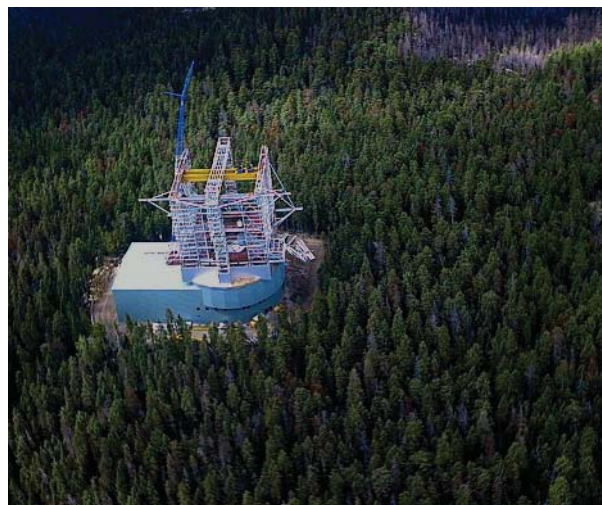
Large binocular telescope during construction, 1999 Mount Graham International Observatory, (University of Arizona)
