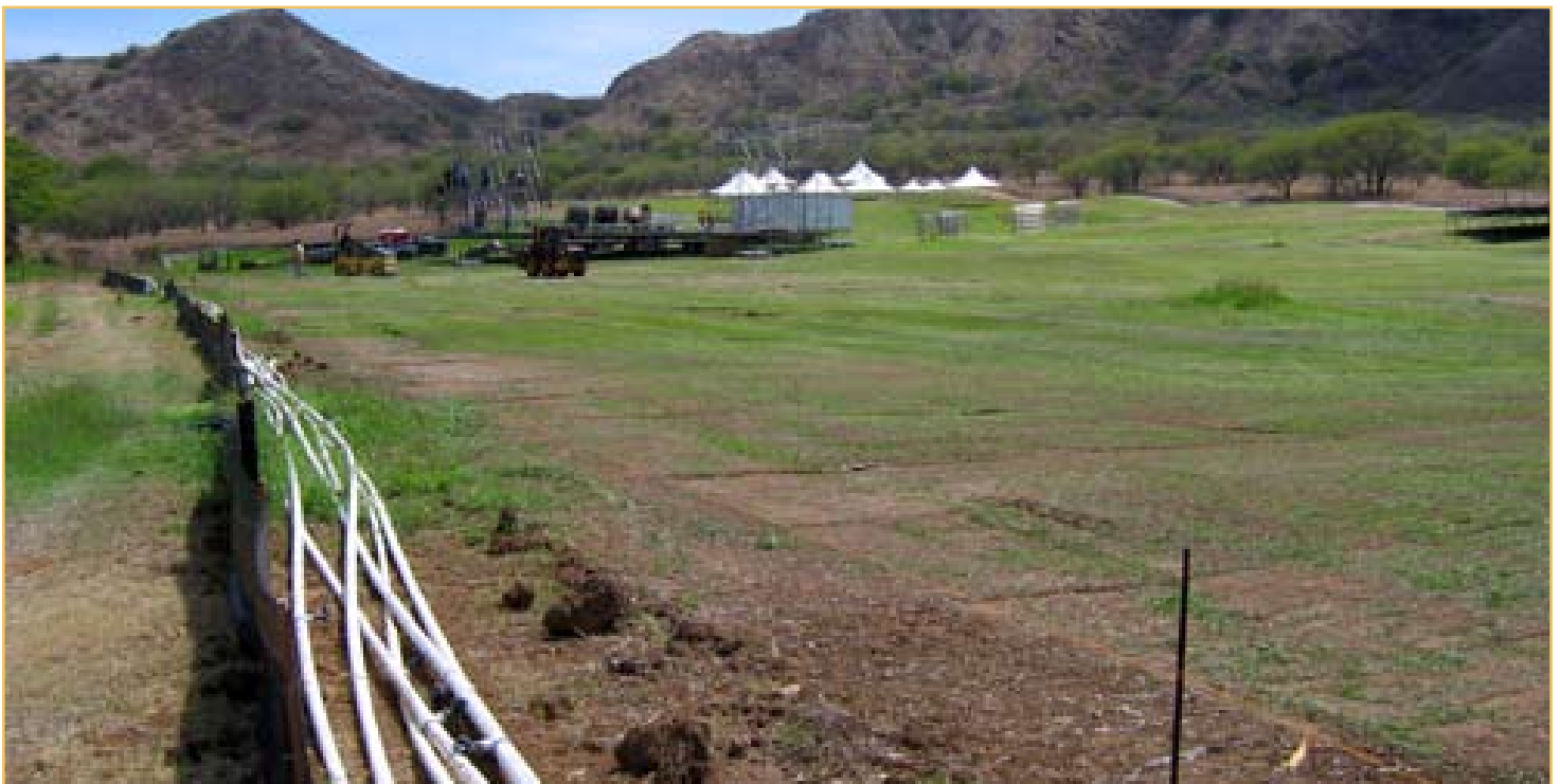
The irrigation lines have been removed and placed along the silt fence.
