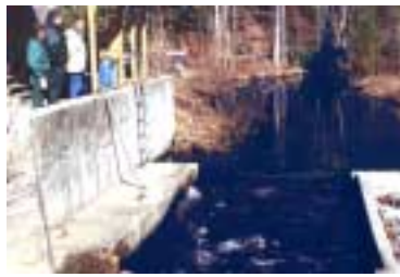
Service personnel examine the Cherokee Tribal Fish Hatchery water intake structure during a visit to the Cherokee Reservation in North Carolina.
