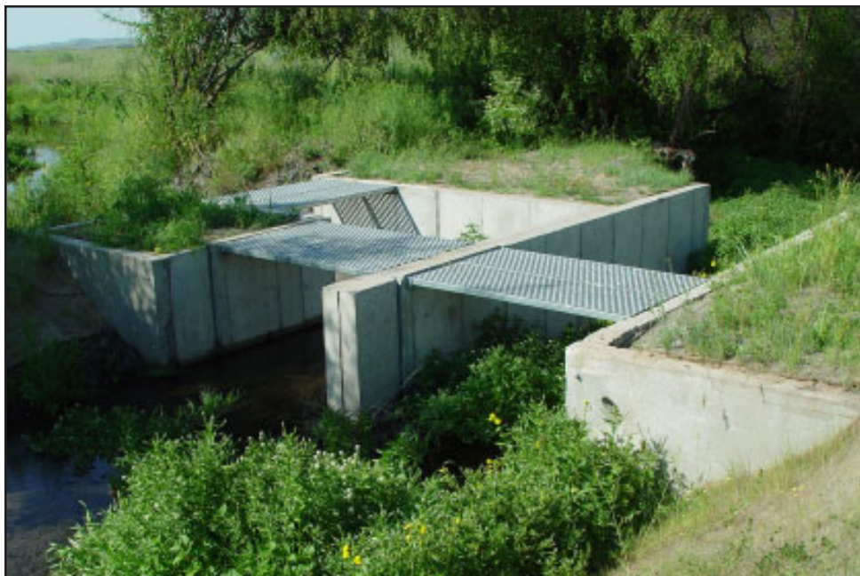
Parker Creek Restoration Project: The water control structure splits the flow of Packer Creek, Washington, between the creek and the rehabilitated wetlands complex. (BLM)
