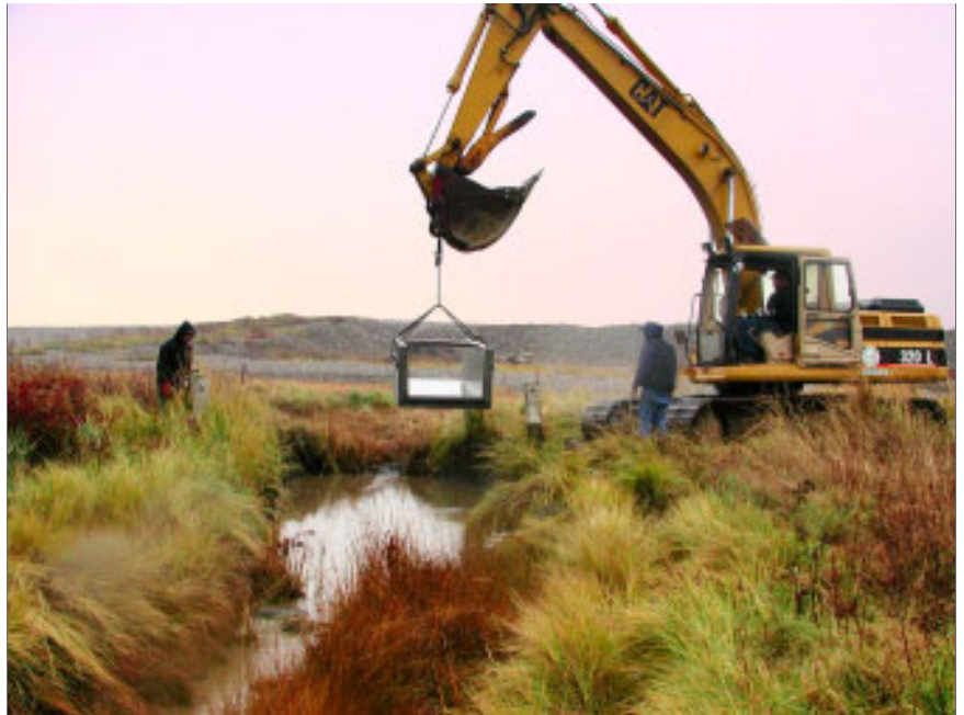
Replacement of an undersized culvert to increase tidal flow to a salt marsh in Rockport, Massachusetts. (NOAA)
