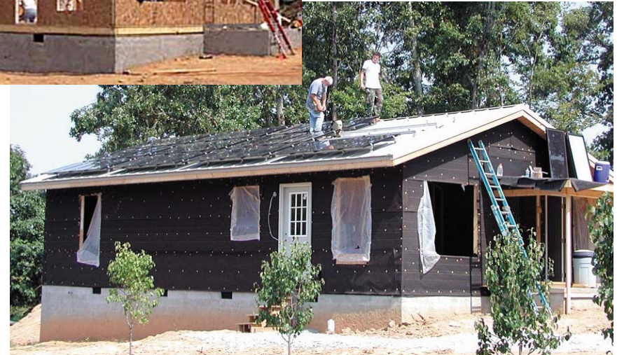
Solar panels on the roof will generate electrical power for the home.
