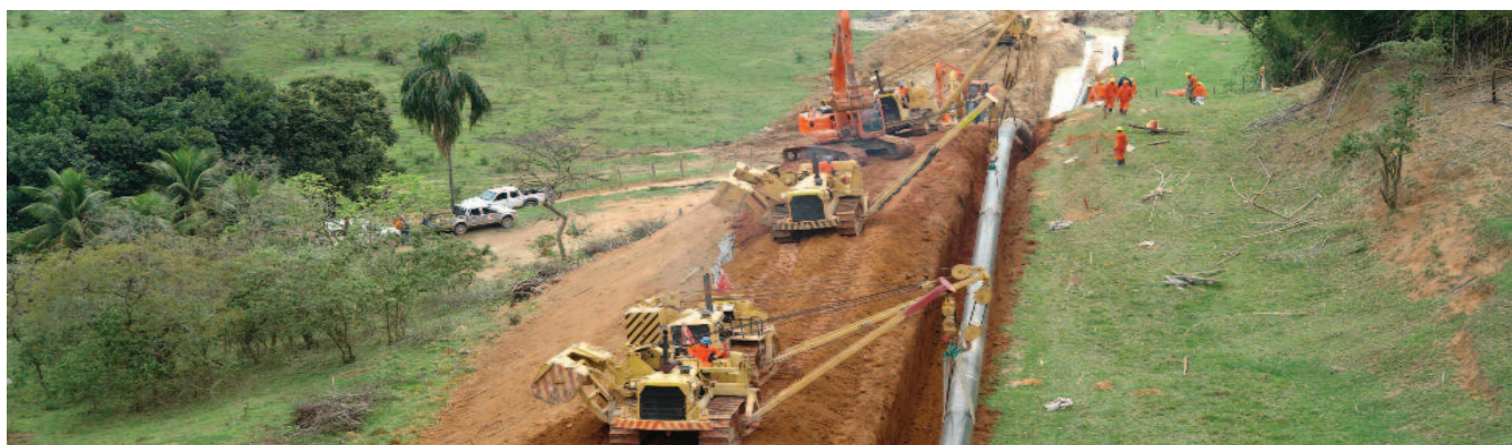
Deployment of pipelines to transport natural gas on a stretch of rising hill, using tube settlers, hydraulic excavators and other heavy equipment.
