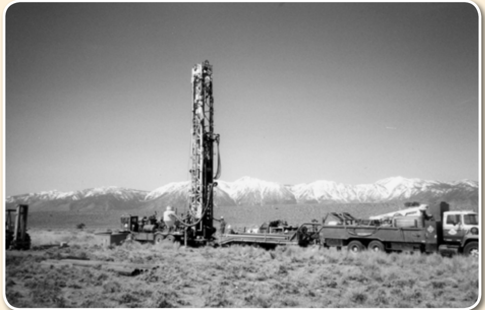
Figure 1: Dresser Model T70W direct-circulation rotary drilling rig using air and equipped with hydraulic accentuated casing hammer. Photo was taken in May 1999 during the installation of two 6-inch diameter 250-ft deep monitoring wells by Beylik Drilling, Inc. (now Layne-Christensen) along the foothills of the Pine Nut Range near Minden, Douglas County, NV. Background – Carson Range east of Lake Tahoe and the Sierra Nevada.
