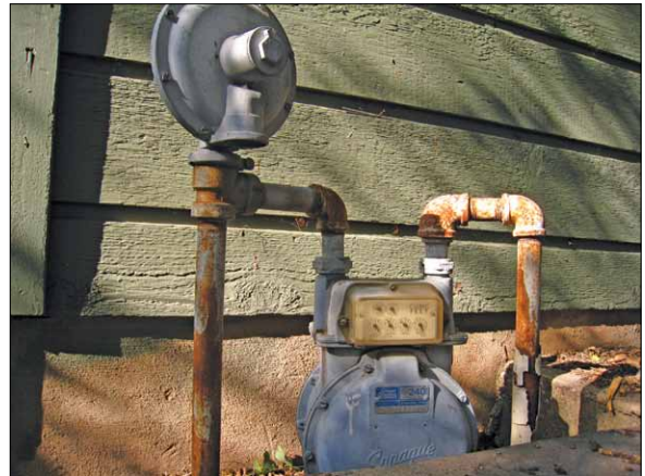
Residential Gas Utility Meter
