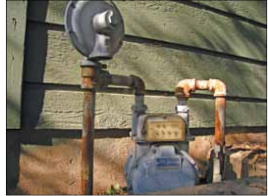
Figure 4-7 Residential Gas Utility Meter
