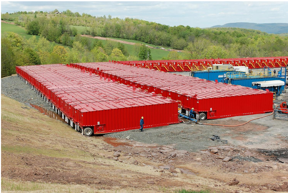
Photo 6.1 - A representative view of completion activities at a recently constructed well pad (New August 2011)
