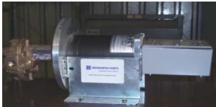
Solar-charged glycol pump (Source: BP)
