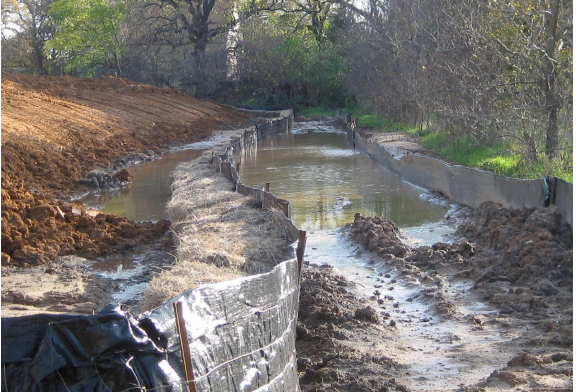
Run-off, Chesapeake Energy pad site, Residential Neighborhood, Ft. Worth Tx.
