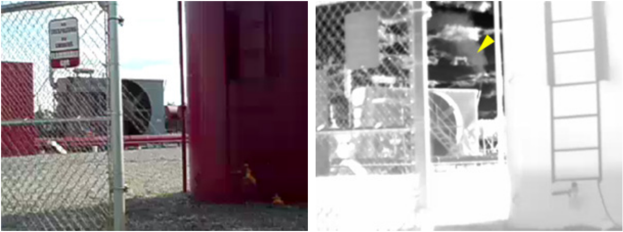
Figure 10: FLIR images of a compressor at the Energy Corp. Compressor Station. Gas emissions from the compressor's packing glands are reference by the yellow arrow.
