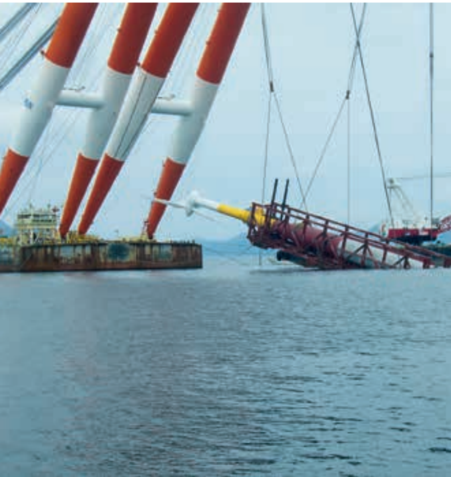
Floating installation, Japan © MOE
