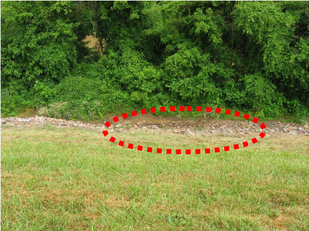
PHOTO 16: WET AREA AT TOE OF SOUTHERN EMBANKMENT OF SECONDARY POND (LOOKING SE)
