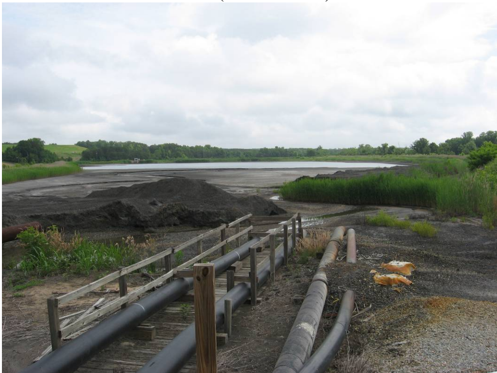
PHOTO 4: SLUICE LINE DISCHARGE AREA AT SW CORNER OF PRIMARY POND (LOOKING NE)
