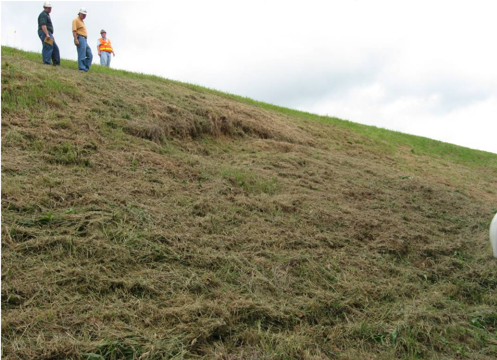
PHOTO 10: SURFICIAL SLOUGH OF PRIMARY POND SOUTHERN EMBANKMENT (LOOKING N)
