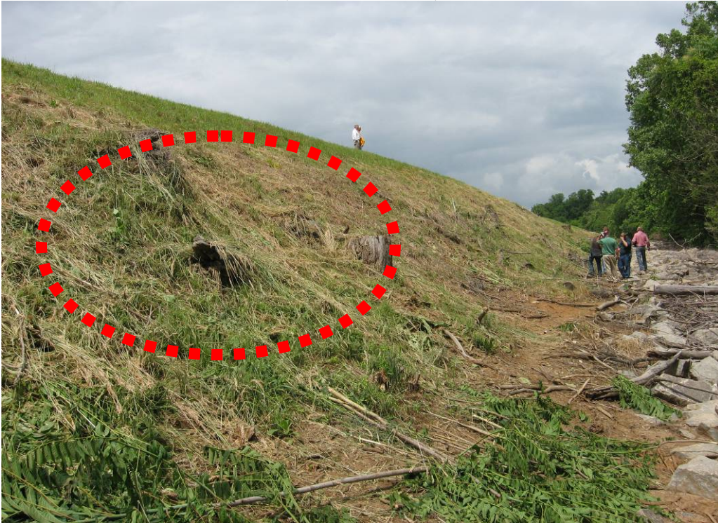
PHOTO 5: STUMPS IN PRIMARY POND SOUTHERN EMBANKMENT SLOPE (LOOKING NE)
