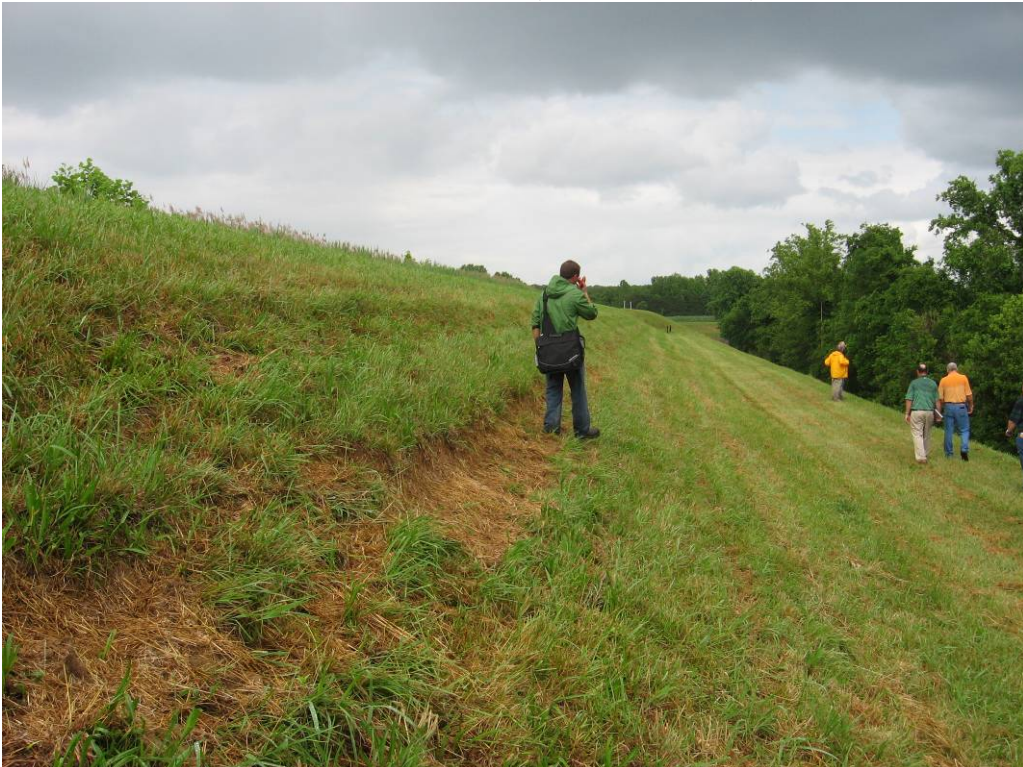
PHOTO 14: RUTTING NEAR CREST OF SOUTHERN EMBANKMENT OF PRIMARY POND (LOOKING NE)
