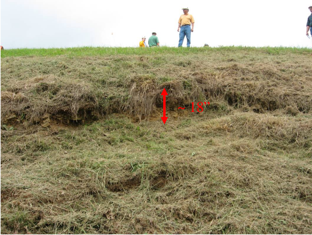
PHOTO 11: SCARP OF SURFICIAL SLOUGH OF PRIMARY POND SOUTHERN EMBANKMENT (LOOKING NW)
