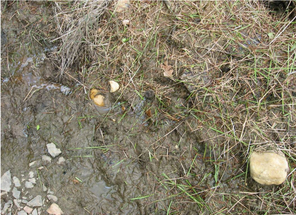
PHOTO 9: SEEPAGE AND SATURATED AREA AT TOE OF PRIMARY POND SOUTHERN EMBANKMENT
