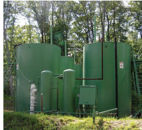
Condensate tanks pull off water from gas and can produce fumes and emissions.
