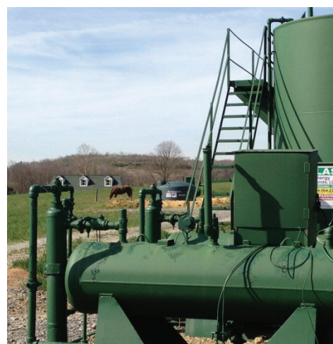
Well equipment close to home.
