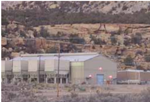
FIGURE I-15. COMPRESSOR STATION Source of NO x .
