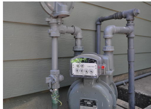
Figure 4-7 Residential Gas Utility Meter
