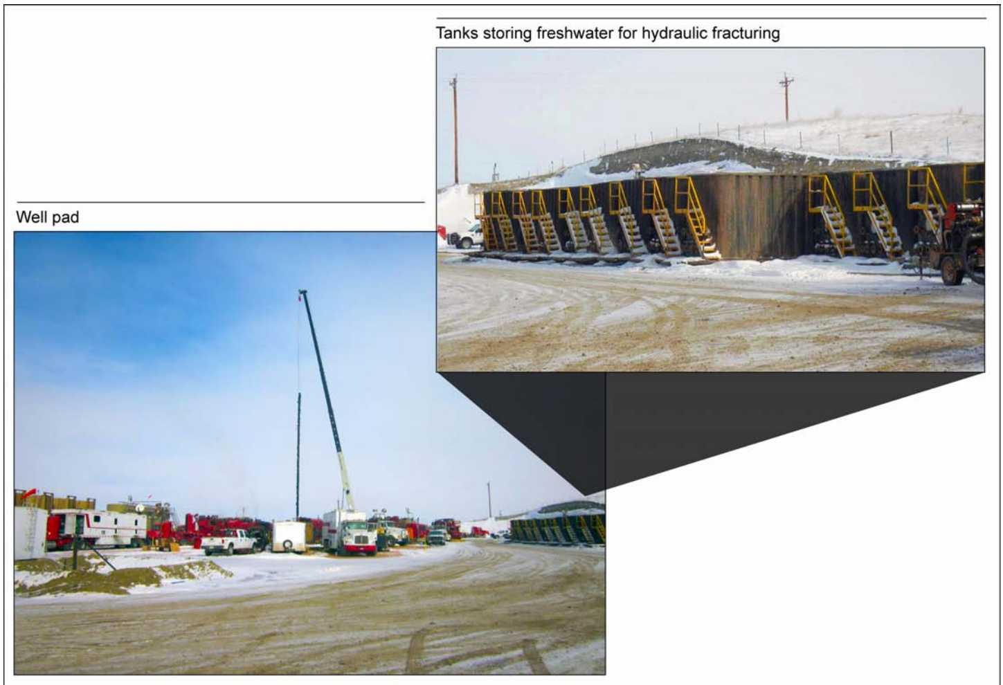
Figure 3: Well Pad and Freshwater Storage Tanks
