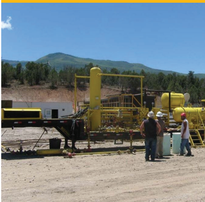
Figure 12: Green Completion Equipment
