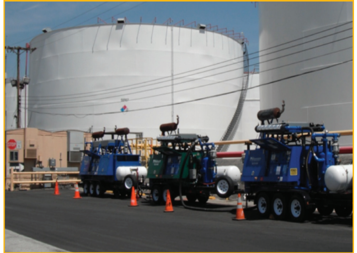
Figure 31: Vapor Recovery Unit
