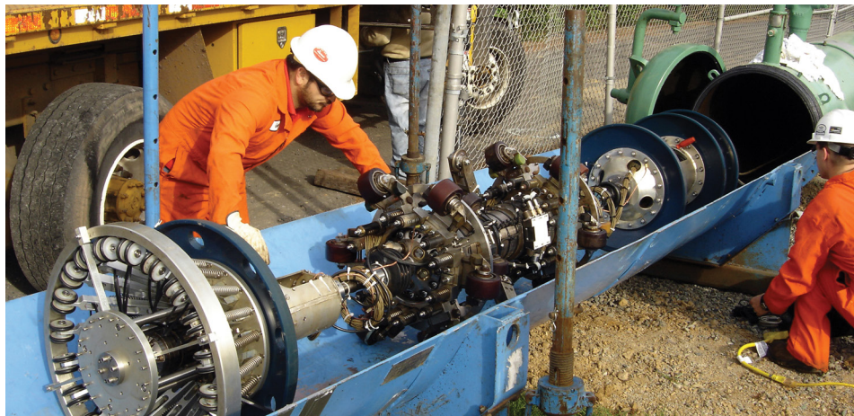
Williams pipeline employees remove an internal inspection device from the pipeline known as a "smart pig."
