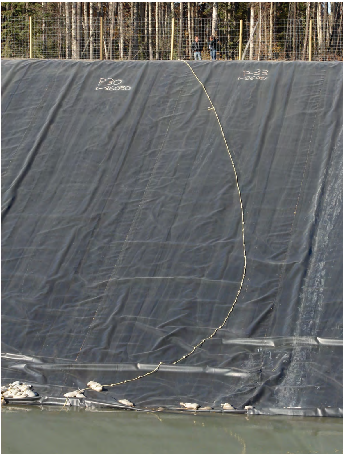
Talisman's leaking storage "pond." Photo – Will Koop
