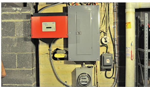
The red box is the inverter
