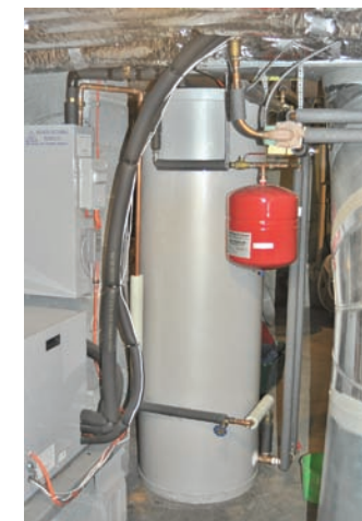
Their hot water tank looks like most hot water tanks, except for the red pressure release tank on the side.
