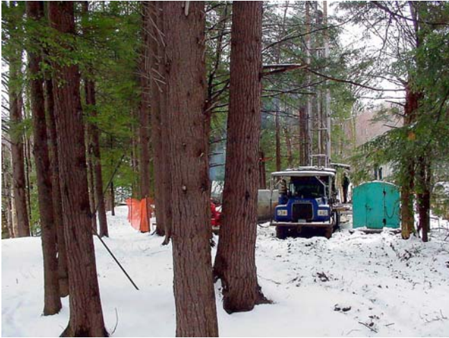
Zoar Well Plugging Site. The construction of the access road and well site was designed to minimize disturbance to the surrounding area.
