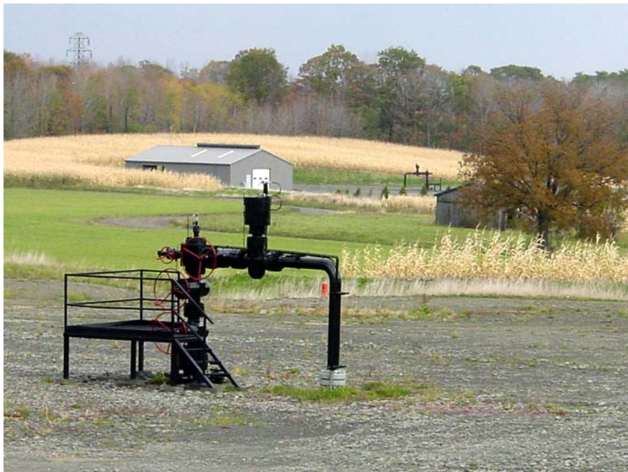
Stagecoach Gas Field, which started operation in 2002, is the easternmost underground natural gas storage field in the US. The field uses innovative horizontal wells to increase gas flow. Well CNYOG W-4 is in the foreground and well W-8 and an equipment building are in the background.
