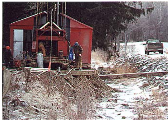
The mostly wooden structure is an older style of drilling rig known as a cable tool rig. It is being used to plug a well in a DOT right-of-way next to a stream.
