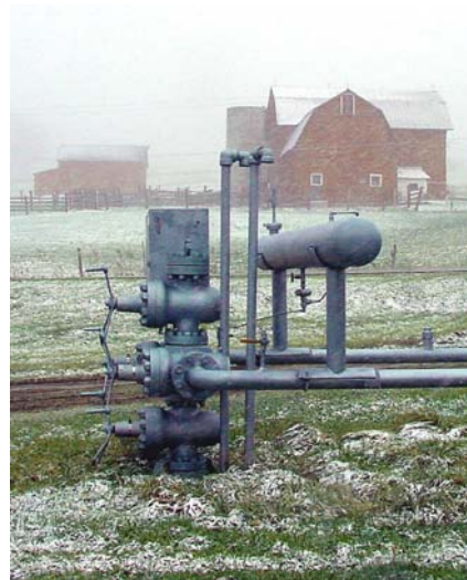
A well at the Woodhull Storage Field in Steuben County. The reservoir has the largest storage capacity in New York.
