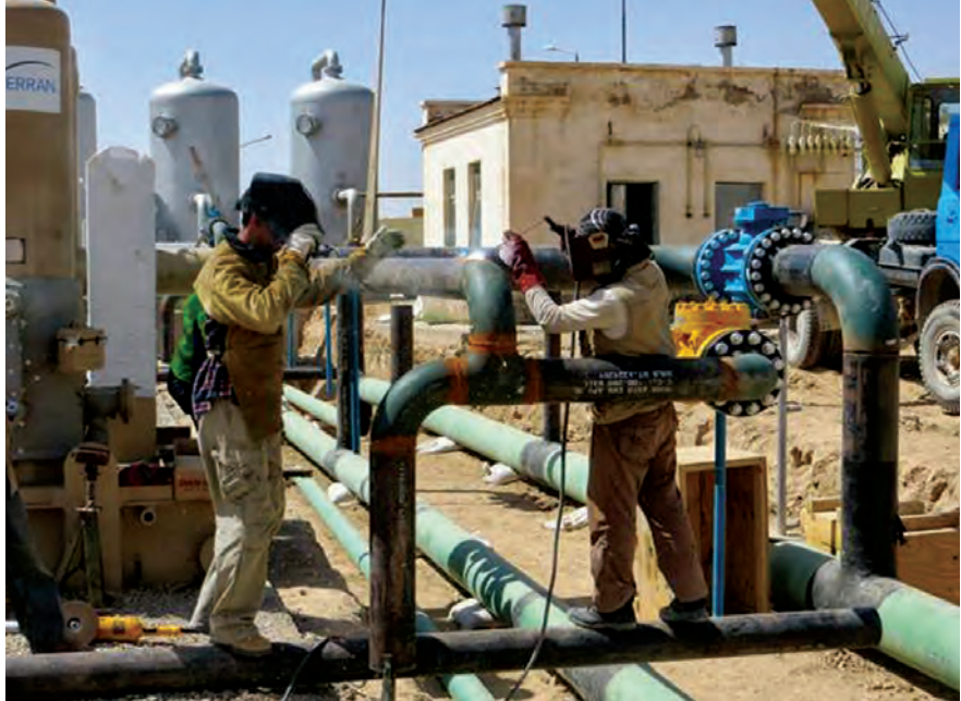
Workers weld a compressor pipe that is part of the Sheberghan pipeline-rehabilitation project. (TFBSO photo)
