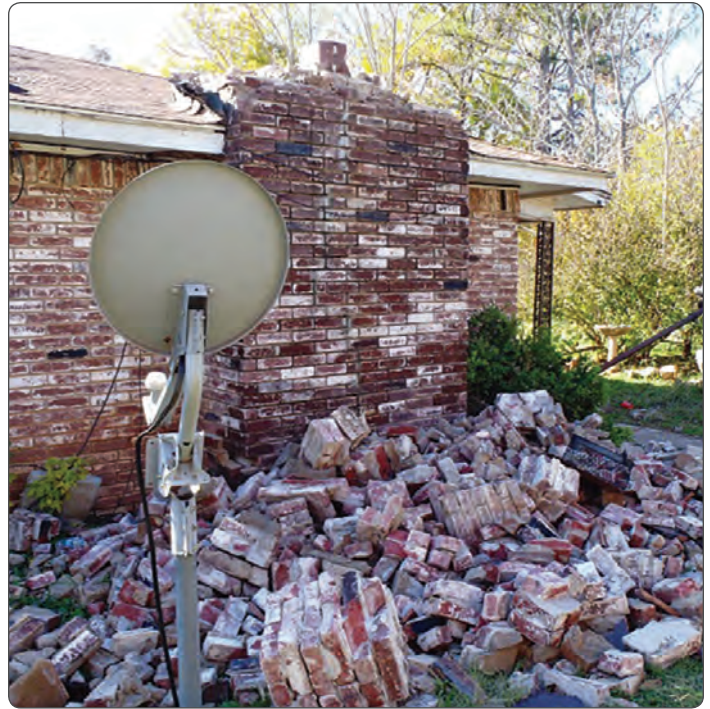
Residential damage from the magnitude 5.7 earthquake in 2011 that struck Prague, Oklahoma. PHOTO BY U.S. GEOLOGICAL SURVEY
