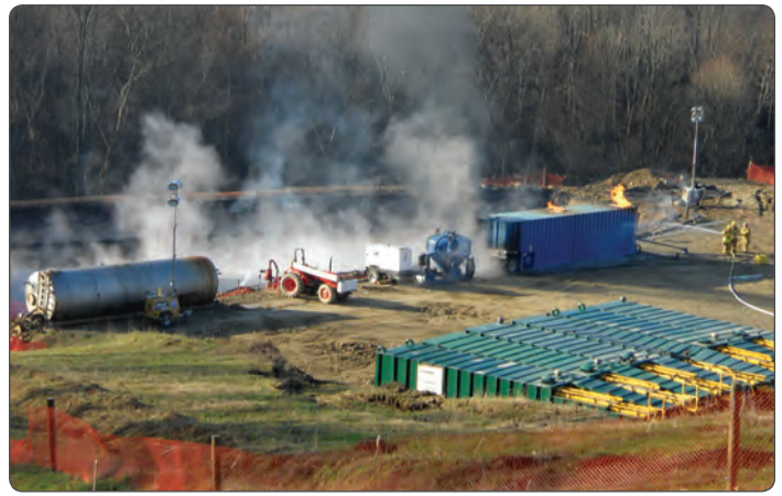
Battling a fracking wastewater liner fire in Hopewell Township, Pennsylvania. PHOTO CC-BY-SA © FRACTRACKER.ORG
