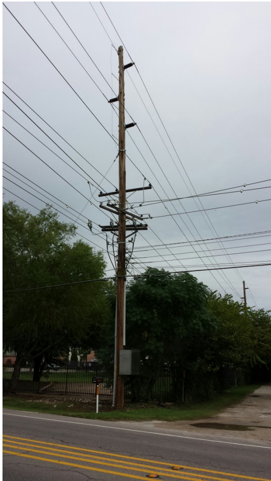
Existing transmission line on property across E McKinney Street from site to the north.
