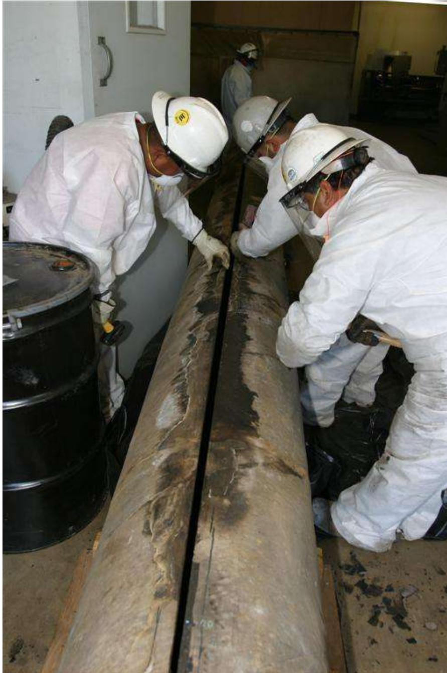
The photograph displays the careful hand removal process of the coating adjacent to the crack.
