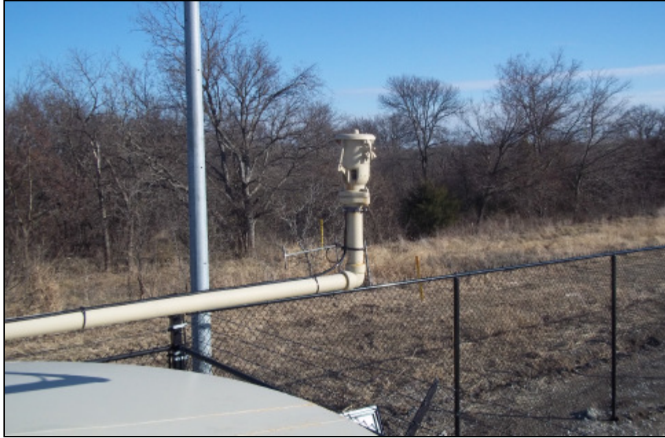
Figure 3.7-3. Storage Tank Vent
