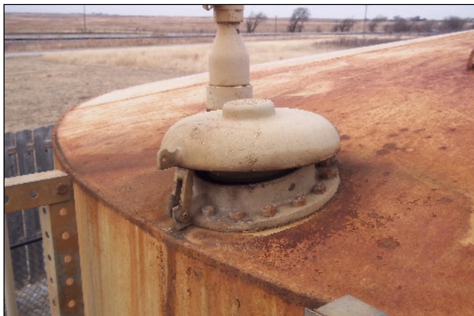
Figure 3.7-1. Thief Hatch Left Open
