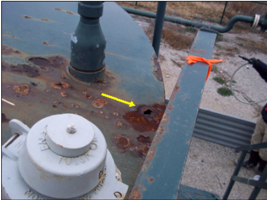
Figure 3.7-5. Hole in Tank Roof - Miscellaneous Emission Source
