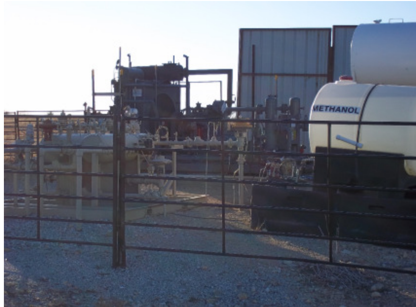
Figure 3.3-7. Site Documentation – Lift Compressor
