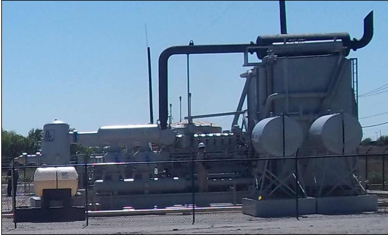
Figure 4.1-3. Natural Gas Compression Engine
