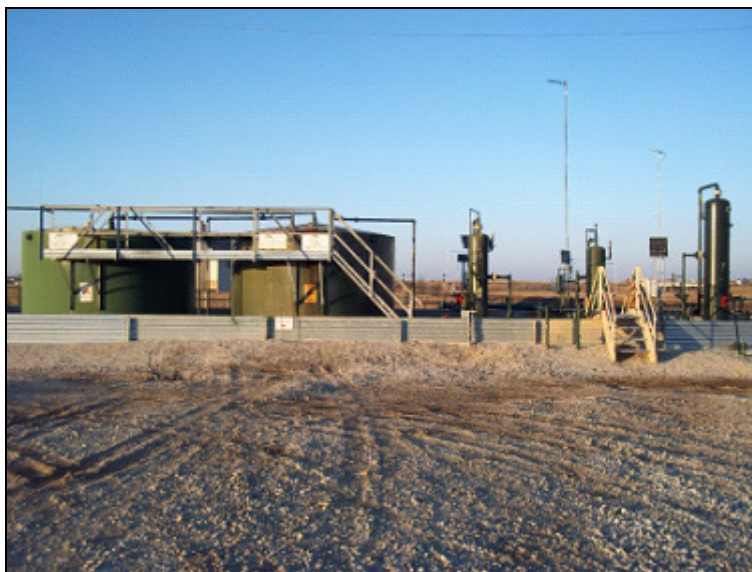
Figure 3.3-6. Site Documentation – Tanks and Separators
