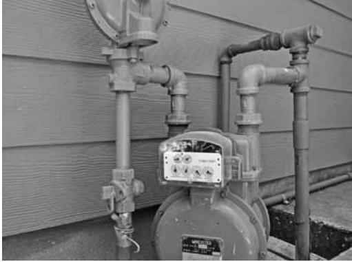
Figure 4-7 Residential Gas Utility Meter
